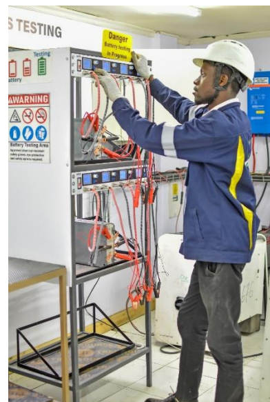
Figure 4 Battery Testing in Progress
