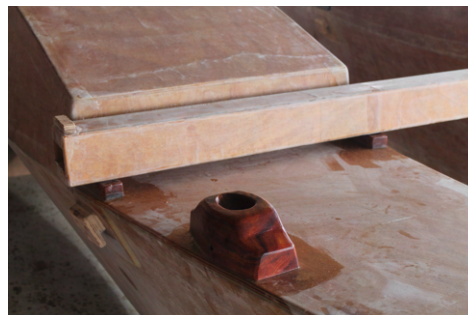
(d) The mast feet are placed on what will later be the outsides (right and left) of the catamaran, so on one hull the mast foot is on the right side, and on the other one the left.
