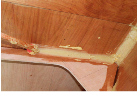
(a) Application of a fillet to the joint of the center bulkhead and the hull side. The tool is easily made by a stick of lumber for the handle and a round plastic piece (e.g. cut from a lid).
