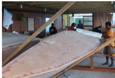
(b) Two layers of glass fiber cloth are rolled over the hull side.
