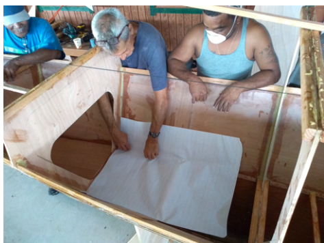
(a) The shape of each bunk-board is different. A large sheet of paper is used to get the hull dimensions right.
