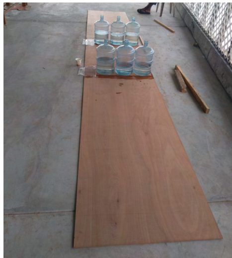
(c) The ply sheets are joined by glued on doublets. Water bottles are used as weight to keep everything in place.
