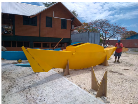
(a) The first hull placed in cradles in front of the slip way
