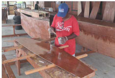
(c) Cabin sides and roof are coated with 3 layers of epoxy (wet-in-wet) as rot prevention.
