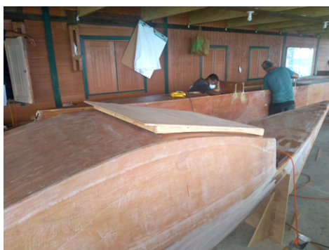
(e) The hatch cover is placed on top of the hatch frame to determine the position for the hinge plates.
