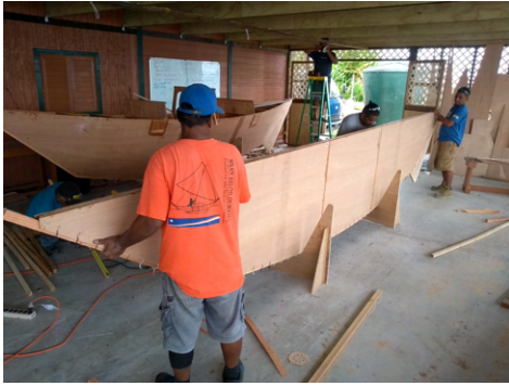
(a) The stitched hull sides are lifted vertically and placed in the cradles.
