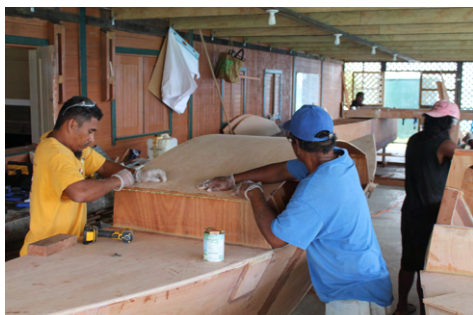
(e) Clamps are used to hold the roof down on the cabin bulkheads (not shown).
