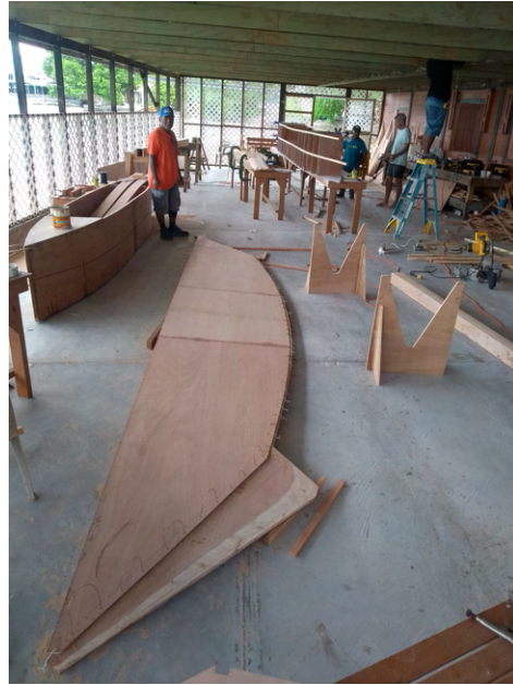
(b) Hull sides, skag, keel and bow are stitched together. Clamps are not necessary anymore. The cradles are already prepared (right) to support the hull shell in its upright position.
