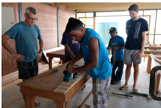
(a) Cut scarf bevels into plywood strips for beams using a planer.
