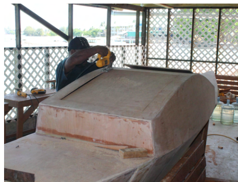
(c) The hatch is cut into the roof after the glue has cured.
