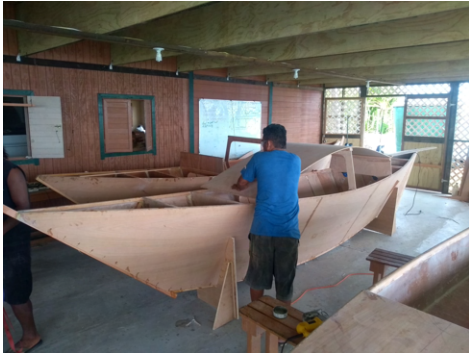
(a) The cabin roof is cut to the width of the bulkhead tops and placed at its desired position.
