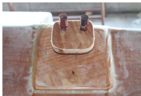
(b) The holes are half filled with slightly thickened resin (like thick syrup). The pins are pressed into the holes, which squeezes out most of the resin.
