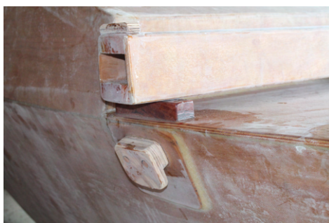
(e) Direct contact between deck and beams would create a narrow gap which would be difficult to maintain and always wet.
