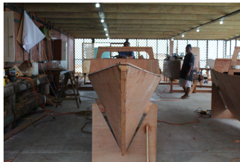
(e) Perfectly aligned deck panels, ready to be glassed on the internal surface.
