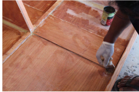
(b) It is very important to cover every bit of bare wood with epoxy to keep the hull rot-free.
