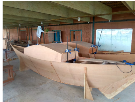
(d) Cabin sides and roof cut to the right dimensions and placed temporarily at the desired positions.
