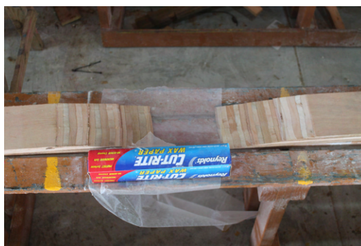
(c) Three scarf joints waiting for glue. Clamps or something heavy will be sufficient to keep them in place until the epoxy has cured. Wax paper is used to separate both joints from each other.
