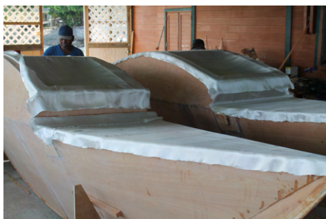
(a) Glass fiber cloth (7 oz. or 180 g) is rolled over the deck and cabin roof.
